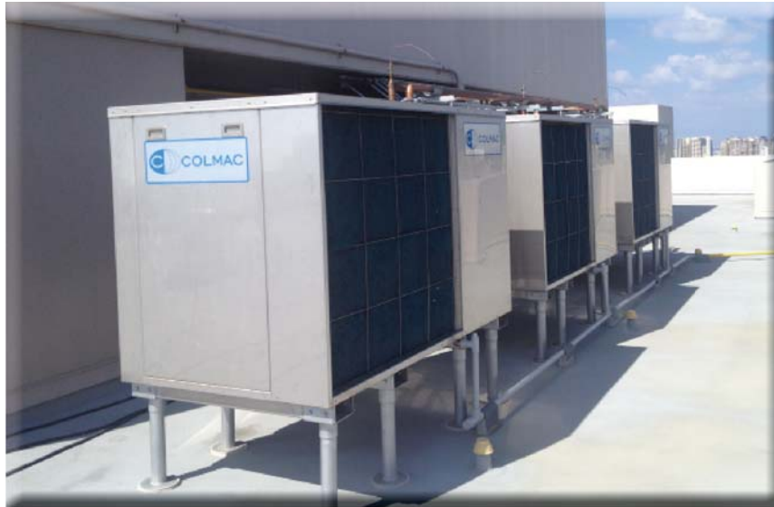
A line of Colmac HPA15 Air Source Water Heating Heat Pumps with RPAF filters on a rooftop in Hawaii
