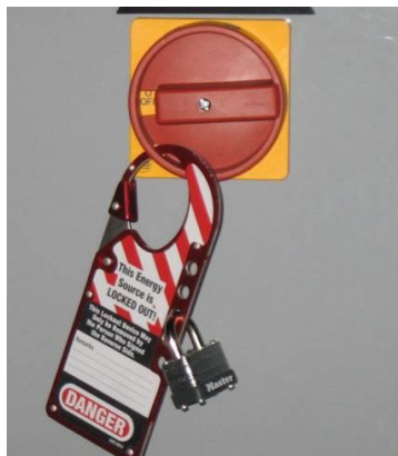
Figure 5: Locked and Tagged Interlock
