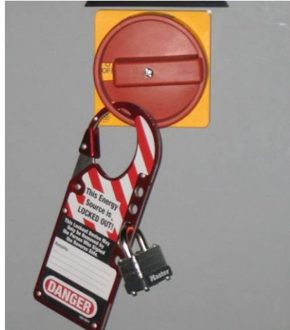
Figure 1: Locked and Tagged Interlock
